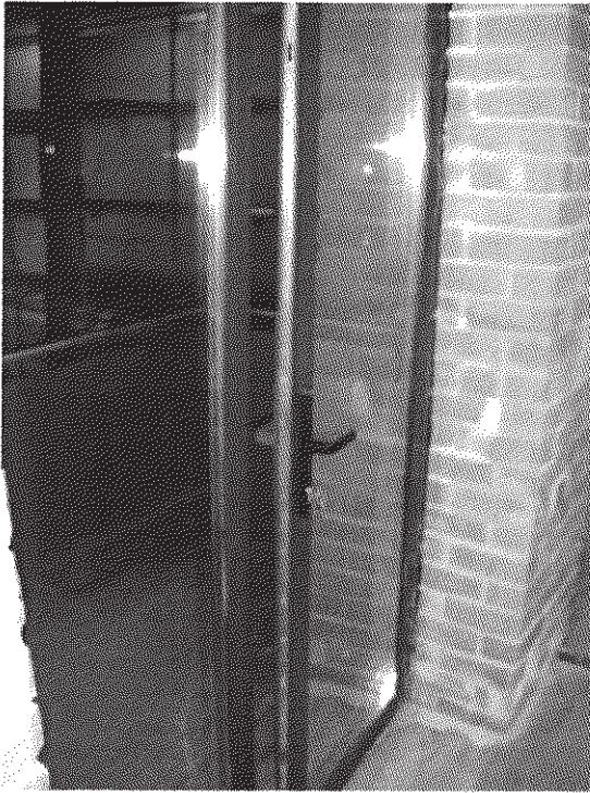
Figure 3: The balcony doors when opened for the ajar measurements to simulate the need for airflow.
